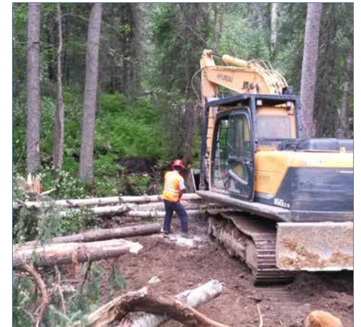
Operating a Chainsaw near heavy equipment -photo by XPLOR2016
